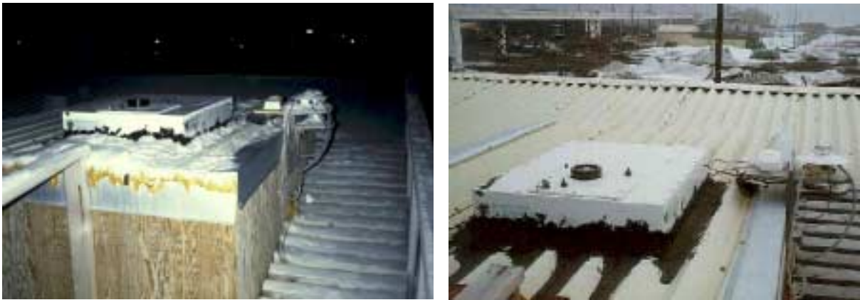
Figure 5.6.1. Roof installation at Barrow during the polar night (left). Note ice buildup on auxiliary sensors (right), and that the collector of the SUV-100, which is heated, remains free of snow, frost, and ice. Same installation during the day (right).
